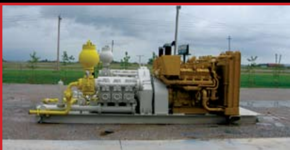
(2) PZ7 PUMP PACKAGES
